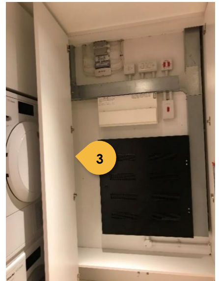
UTILITY ROOM (5F)
